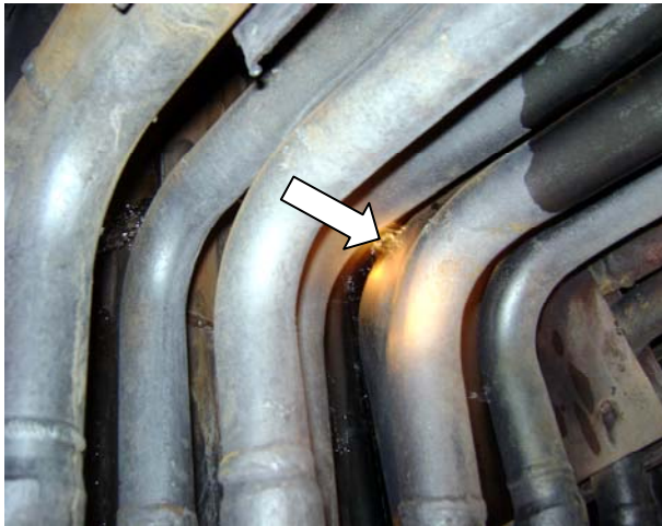
Case 5: The SH coil bends had come close to the casing, that the bends had got eroding. The shields were not placed properly during a maintenance & it led to failure of SH.
