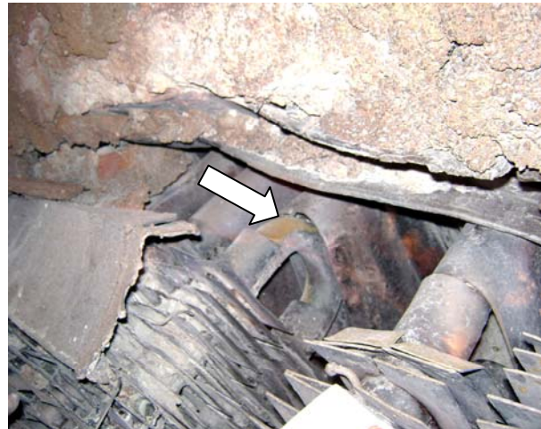
Case 6: The protection shield at bends was not placed properly during maintenance. This had led to a stoppage of the plant. There is a gas baffle to prevent the gas going along the bends.
